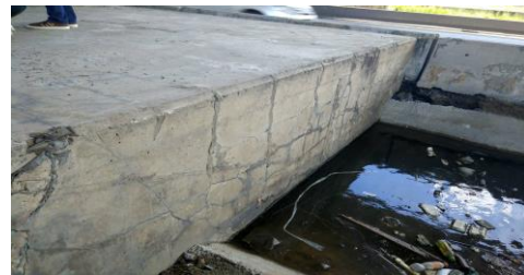
Fig.1 Cracking of a concrete foundation in Thailand
