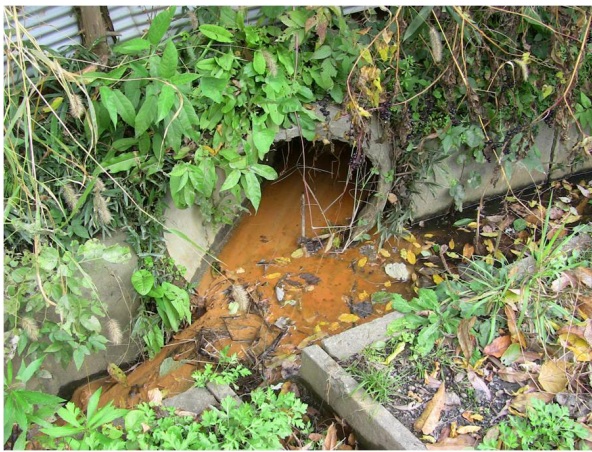
Figure 2 Leachates at the sampling point for VI landfill
