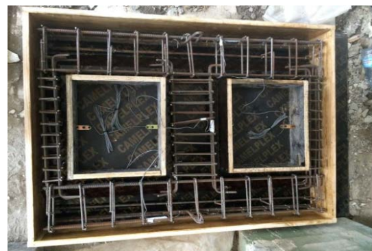
Fig.4 The formwork, reinforcements, and opening locations layout for a typical wall panel [16]
