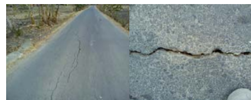
Fig. 2 Typical cracks of the pavement that were built on the residual soil of Lidah Formation in the North East Java
