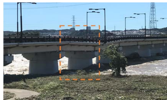
Fig. 1 Example of medium-scale damage
