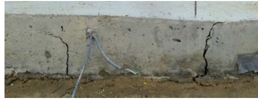
Fig.13 Detail of slab with crack
