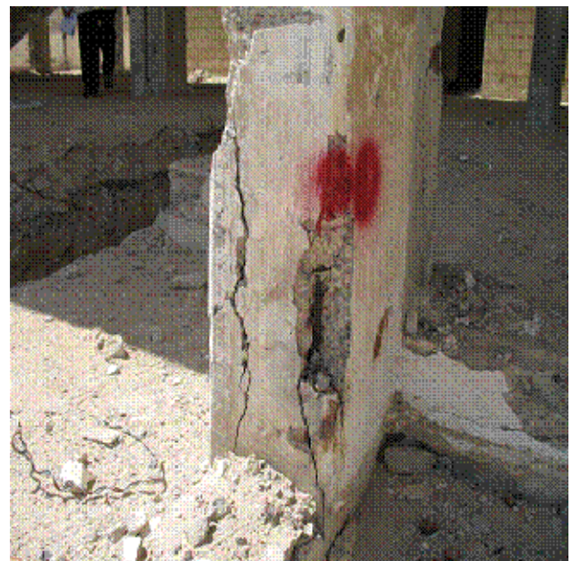
Fig. 7. Exposed corroded reinforcement and expelled concrete at the bottom of a ground floor column.
