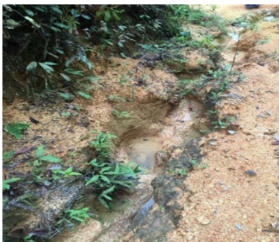
Fig.2 Development of gully nearby transmission tower
