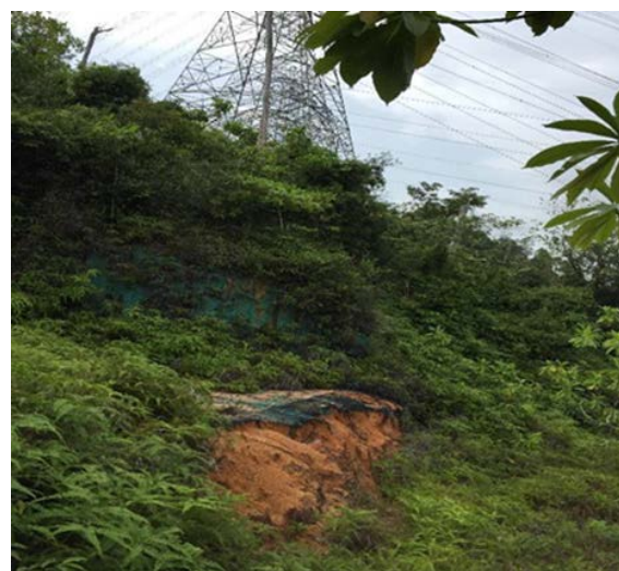
Fig.1 Soil erosion near transmission tower
