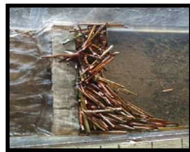
Fig.9 Top view of trapped pieces at box culvert bridge
