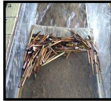
Fig.8 Back view of piece accumulation at box culvert bridge
