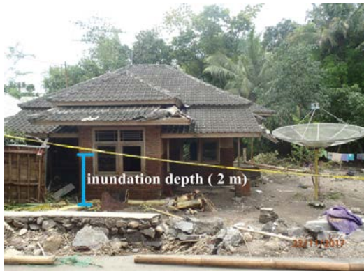
Fig.11 Inundated house near the pipe culvert bridge
