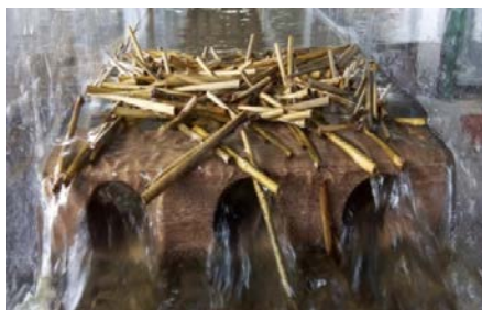
Fig.6 Front view of piece accumulation at the pipe culvert bridge
