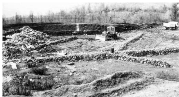
Fig. 4 Rudimentary leachate drainage system in presented case study
