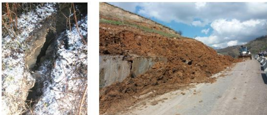
Fig.2 Initial cracks on the slopes and slide bulks on the roads at the root of Kok Tobe
