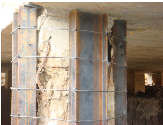
Figure 4. One of buckled basement columns
