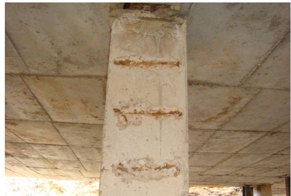
Figure 5. Corrosion of reinforcement of basement slab and columns
