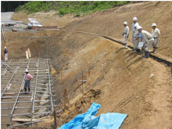
Photo 4 Erosion occurring on 1:1.0 (V:H) Temporary Cut Slope
