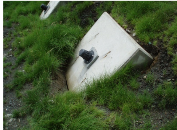
Photo 7 Photograph of Anchor Bearing Plate Indicating Creep Movement of Slope
