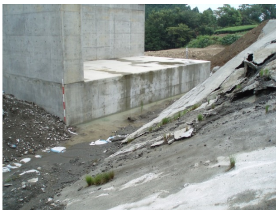
Photo 3 Damage to Temporary Slope Mitigation Works Prior to Permanent Works
