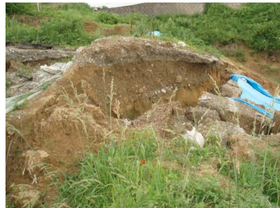
Photo 2 Slope Failure Triggered by Excavation
