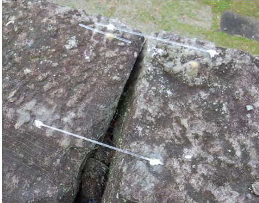
Fig.11 Glass rods for monitoring displacement between stones
