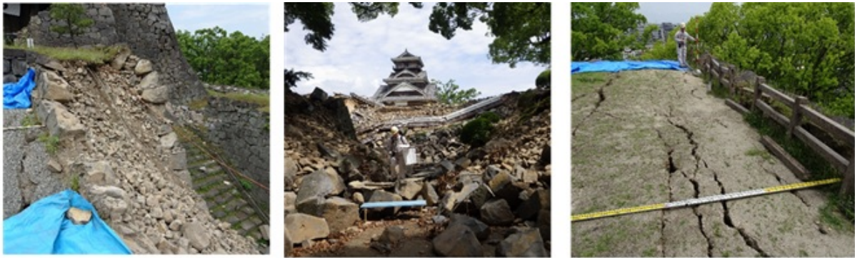
(a) Northern part of castle tower (b) Hooate gate (c) Northern part of Nagatsubone tower
