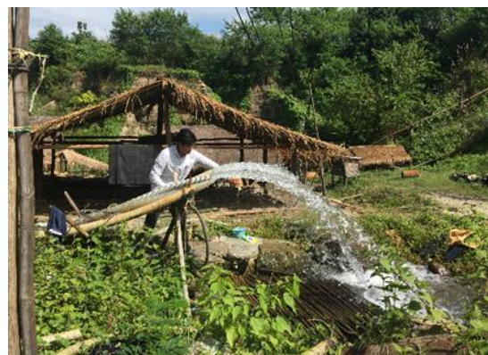
Fig. 2 Groundwater leaked from the tunnel
