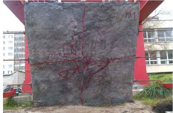
Fig. 4 Cracks on the lower surface of experimental post-tensioned slab after its broken
