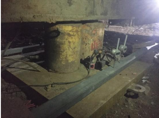
Fig. 4 Equipment underneath platform
