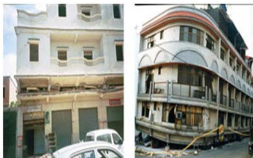
Fig.14 Soft story type progressive collapse occurs on ground floors in 3rd World countries (Hoodline San Francisco 28 February 2016)
