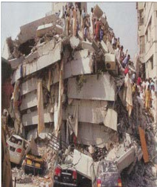
Fig.2 RC Pakistani building earthquake damage resulting in a pancake type collapse (Mother Nature Network)
