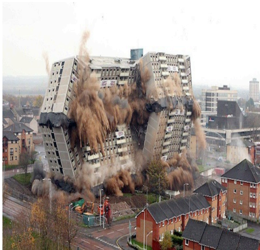
Fig.6 Building showing typical inward falling domino type progress collapse (Demolition Implosion Miami Fort Lauderdale Florida October 1994)
