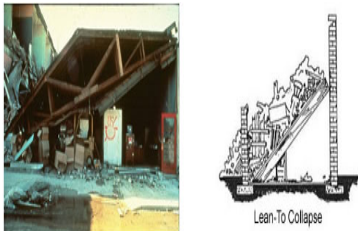
Fig.13 Lean-to type progressive collapse resulting from an earthquake or an uncontrolled demolition (Bomb Attack) (Reid Middleton 8 October 2013)
