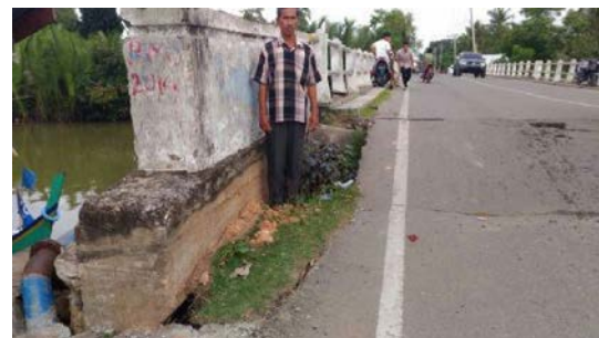
Fig.3 Settlement on the road in Pidie 2016
