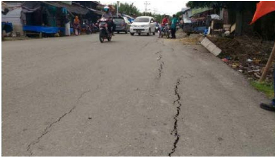
Fig. 7 Cracks on road in Pidie 2016
