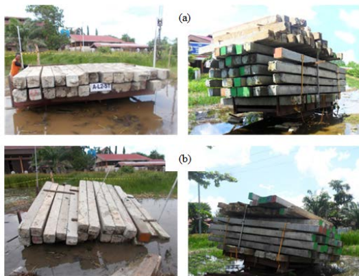
Fig.4. Field loading tests: a) loading on the single pile and pile group; b) after ultimate load conditions were achieved.
