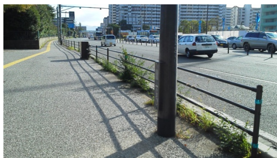
Fig. 1 Some plants established in curbside cracks of road.
