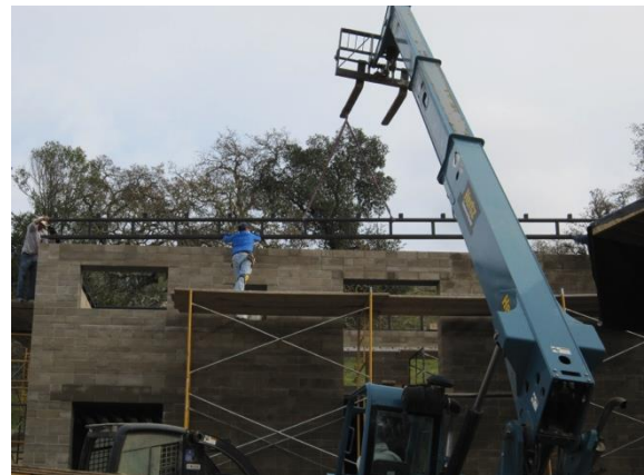
Fig. 5 Watershed Materials' demonstration house under construction in the Bay Area of California. Photo by David Easton
