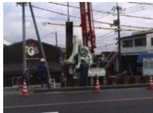
Photo. 5 Working scenery in which WSFRM was used in the pulling-out of a steel sheet-pile
