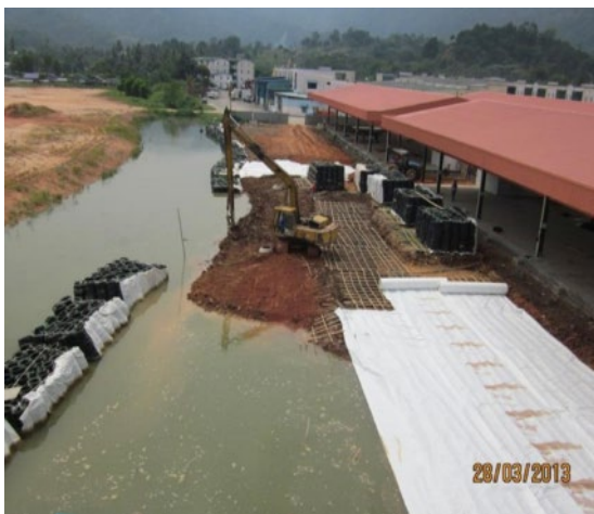
Fig.10 Houses to be built over soft peat devoid of foundation but supported on 'geobamtile' system [48]
