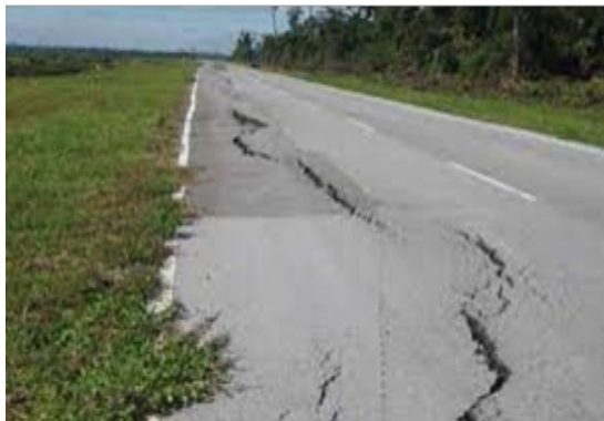
Fig.5 Failure Road on Kg Sungai Bidut, Sarawak Road [30]
