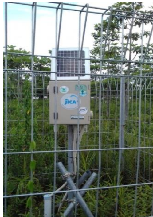
Fig 1. Photo of the SESAME equipment installed on peatlands
