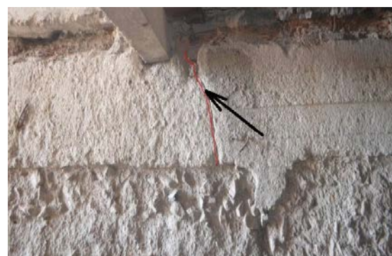
Fig. 1 Cracks in the foundation
