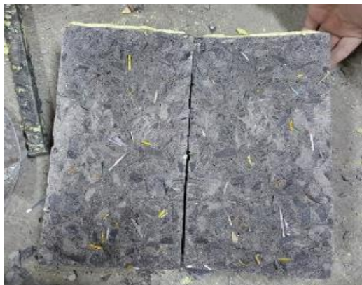
Fig. 10 Fiber sticking out of concrete surfaces.
