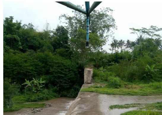
Fig.5 The acoustic sensor of the Kopen AWLR Station
