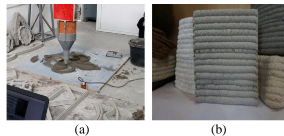
Fig. 3 Printing a small-scale architectural structure with the S-6045 3D printer: (a) printing process and (b) type of layers in the finished product
