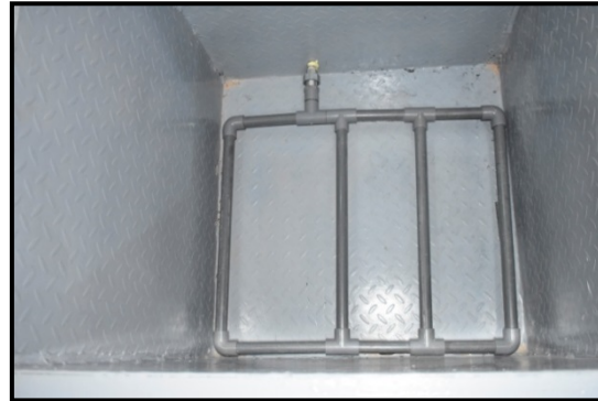
(a) water distribution panel
