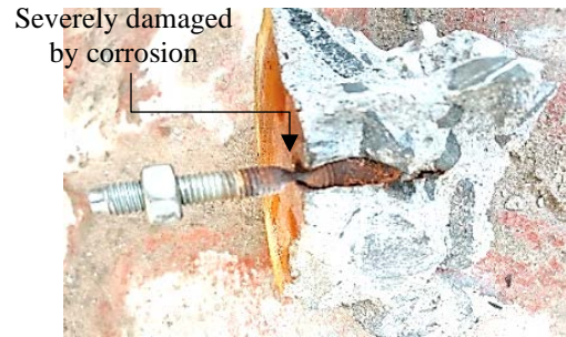
Fig.17 Concrete Cone failure of Corroded Expansion Stud Anchor bolt
