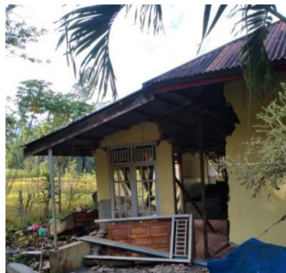
Fig. 2 One of the heavily damaged homes owned by inhabitants of Nagari Kajai (0°09'48.0"N & 99°55'50.1"E).
