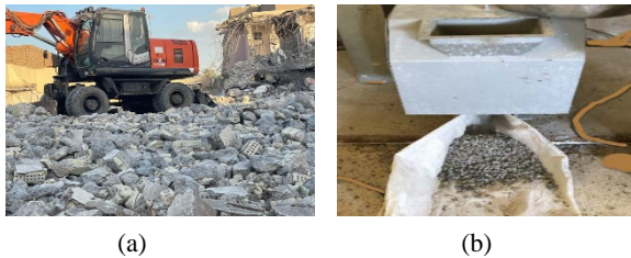
Fig.1 Buildings in Iraq after demolition. a. demolition of an old building. b. grinding of crushed concrete.
