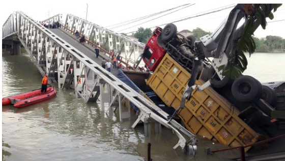
Fig.2 Photo of the collapsed span (documentation of Directorate for Eng. Affairs of Roads and Bridges, Ministry of Public Work and Housing, Indonesia)
