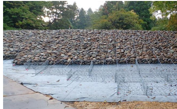
(a) Front view of the downstream slope partially placed by the gabion mattresses and covered with the non-woven geotextile sheet
