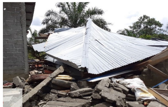
Fig.1 URM hollow brick house damage due to the 2022 West Pasaman Earthquake
