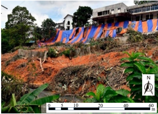
Fig. 2 A photo of the affected area taken two days after the landslide (Source : The Sun)
