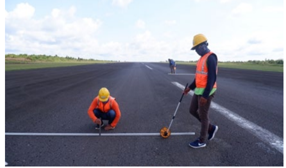
Fig. 4 Rutting measurements on TJQ runway
