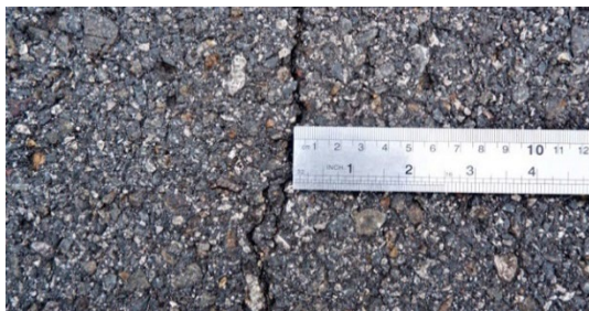
Fig. 7 Crack measurement on PKY runway
