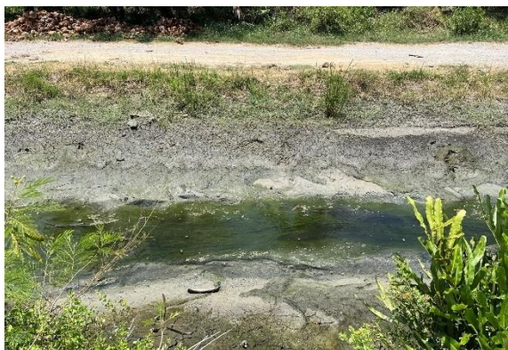
Fig. 1 Sediments in drainage canal
