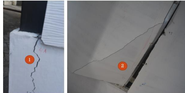
Fig.31 Sheathing damage at 40 kN: bigger plaster cracks and screws are taken out
