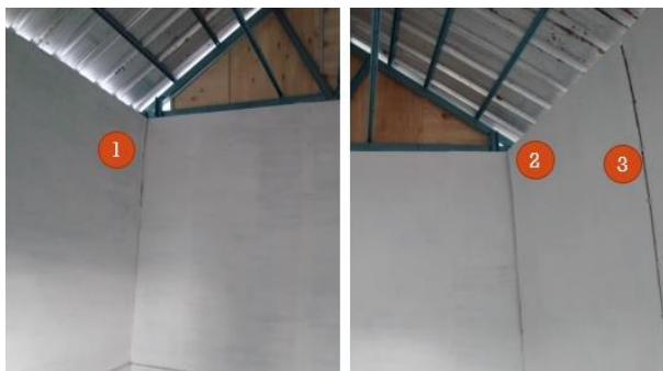
Fig.30 Sheathing damage at 30 kN: more screws on the wall were pulled through the GRC
