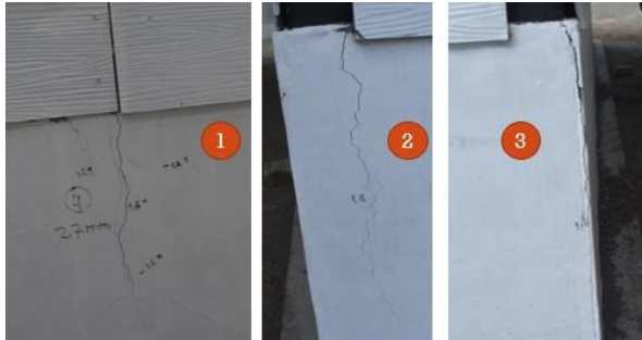
Fig.29 Plaster cracking damage at 20 kN: the plaster starts hairline cracks at the column
