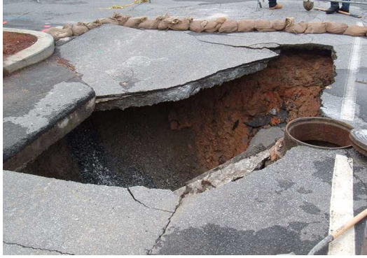
Fig. 1 Occurrence of sinkhole in pavement.
