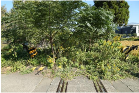
Fig 7 Tracks of another railway without vegetation management after the Kumamoto Earthquake
