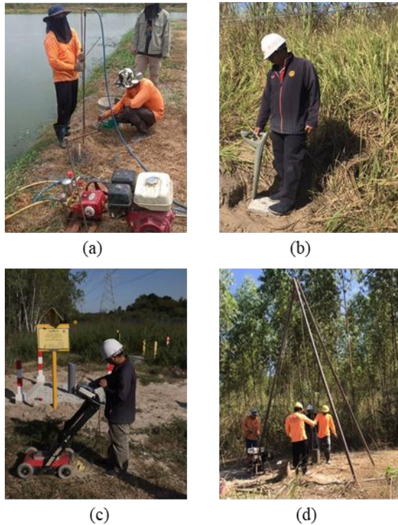
Fig. 4 SUE field operations: (a) water jetting for physical verification of pipeline location and depth; (b) utility detection using Radiodetection RD4000 electromagnetic locator; (c) GPR survey using MALA Easy Locator; (d) soil sampling at test location.
