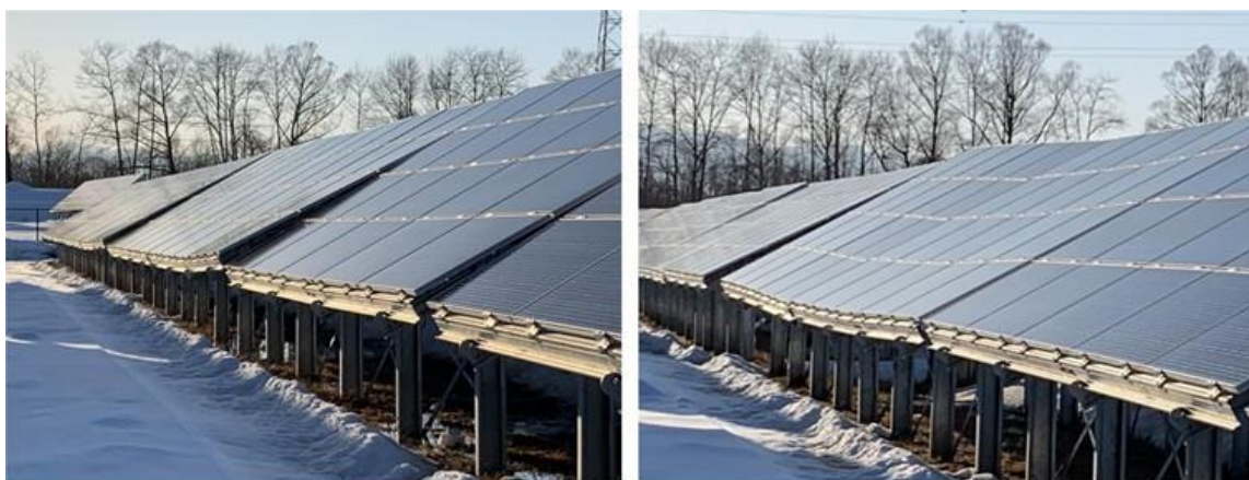
Fig. 1 Examples of frost heave damage to solar panel mounts observed in eastern Hokkaido.
