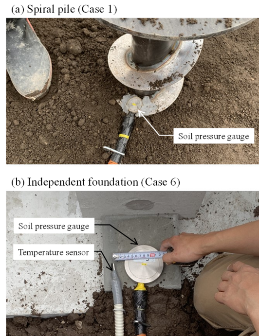
Fig. 8 Installation of soil pressure gauges on the spiral pile and independent foundations.
