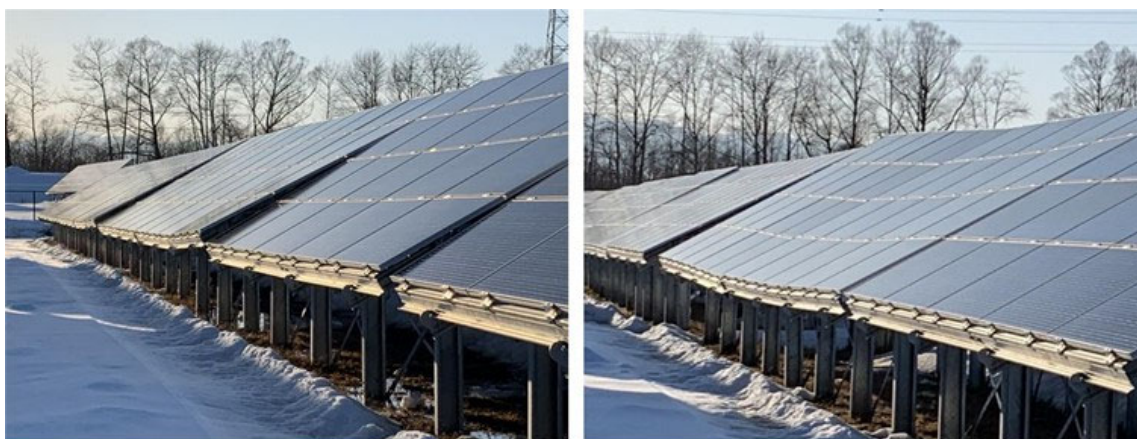
Fig. 1 Examples of frost heave damage to solar panel mounts observed in eastern Hokkaido.
