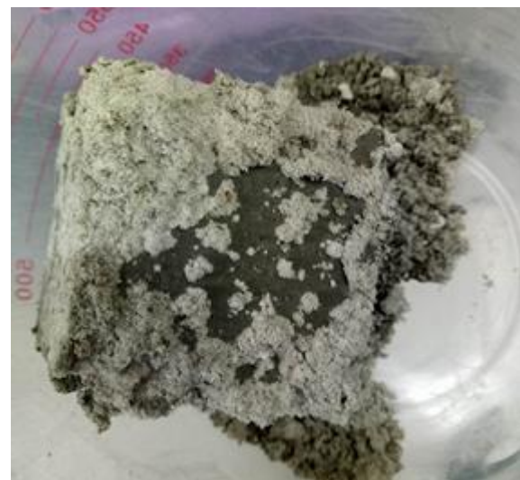
Fig. 4 Occurrence of Efflorescence
