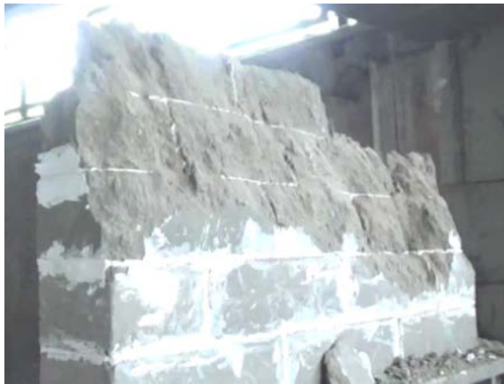
Fig. 6 Complete failure of unreinforced wall
