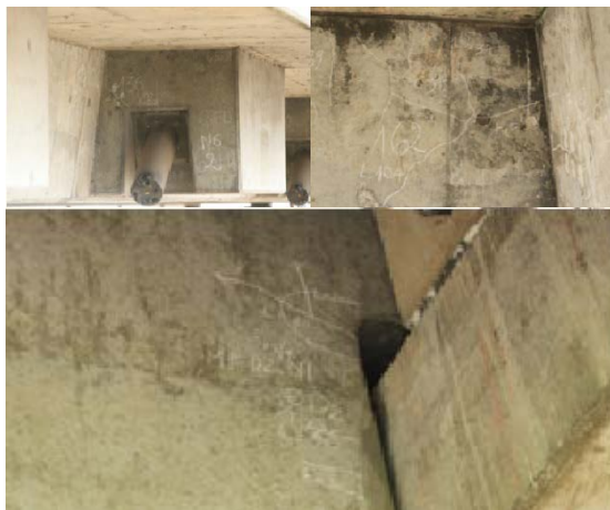
Fig. 2 A lot of cracks were found on the My Thuan bridge: a - the cable to plate fixing area, b - a connection between the crossbeam and deck slab, c
