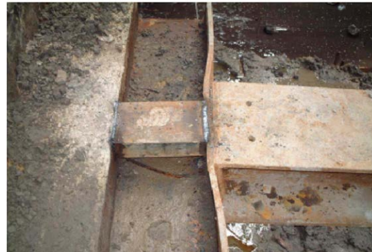
Fig.10 Buckling of walers [7]
